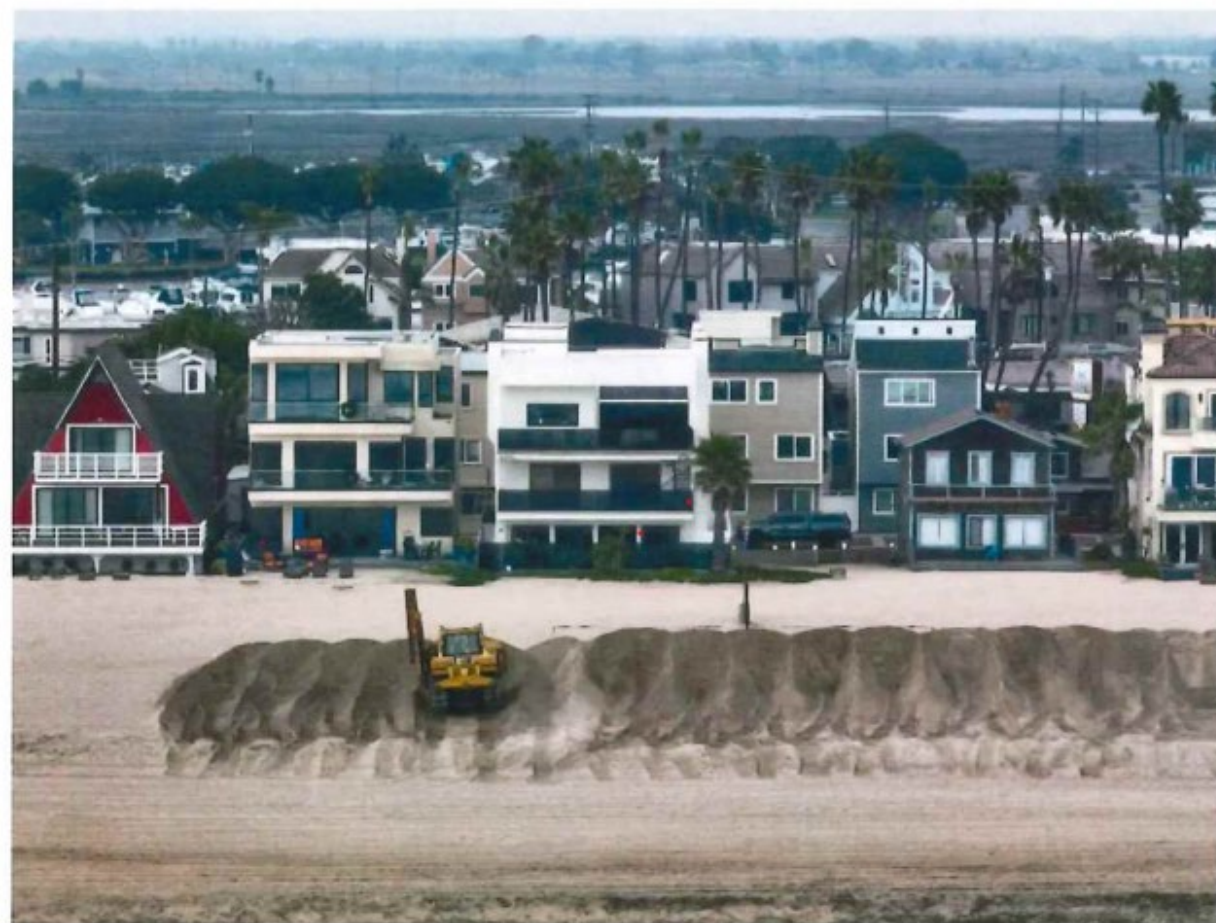
A worker builds a sand dune ahead of an incoming storm at Surfside on Monday, December 13, 2021. The Surfside-Sunset Sand Nourishment project is expected to start Fall 2024. (Photo by Jeff Gritchen, Orange County Register/SCNG)
